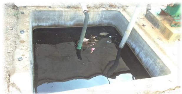
Fig 1 Landfill leachate collection tank
