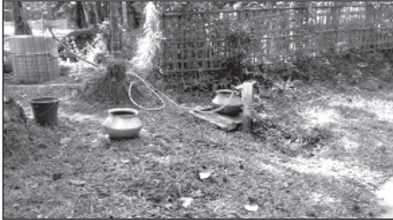
Water supply connection at Dhuptali (Kuki Bari)
