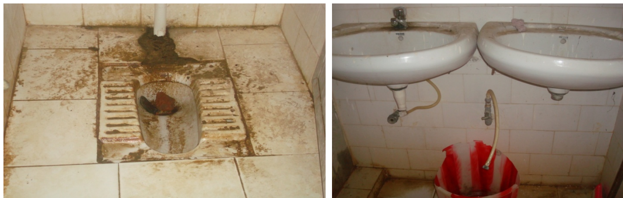
Condition of Latrine & Basin at EMRS, Bhawanipur
