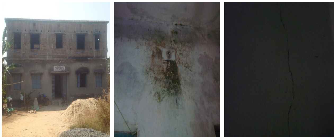
Condition of the half constructed building and walls of the staff quarters of EMRS
