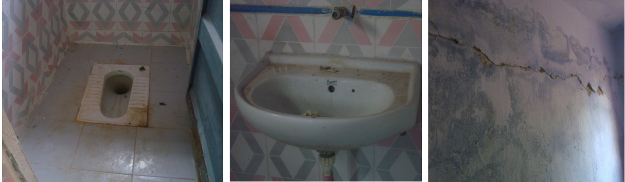
Condition of Latrine and Basin in the EMRS
