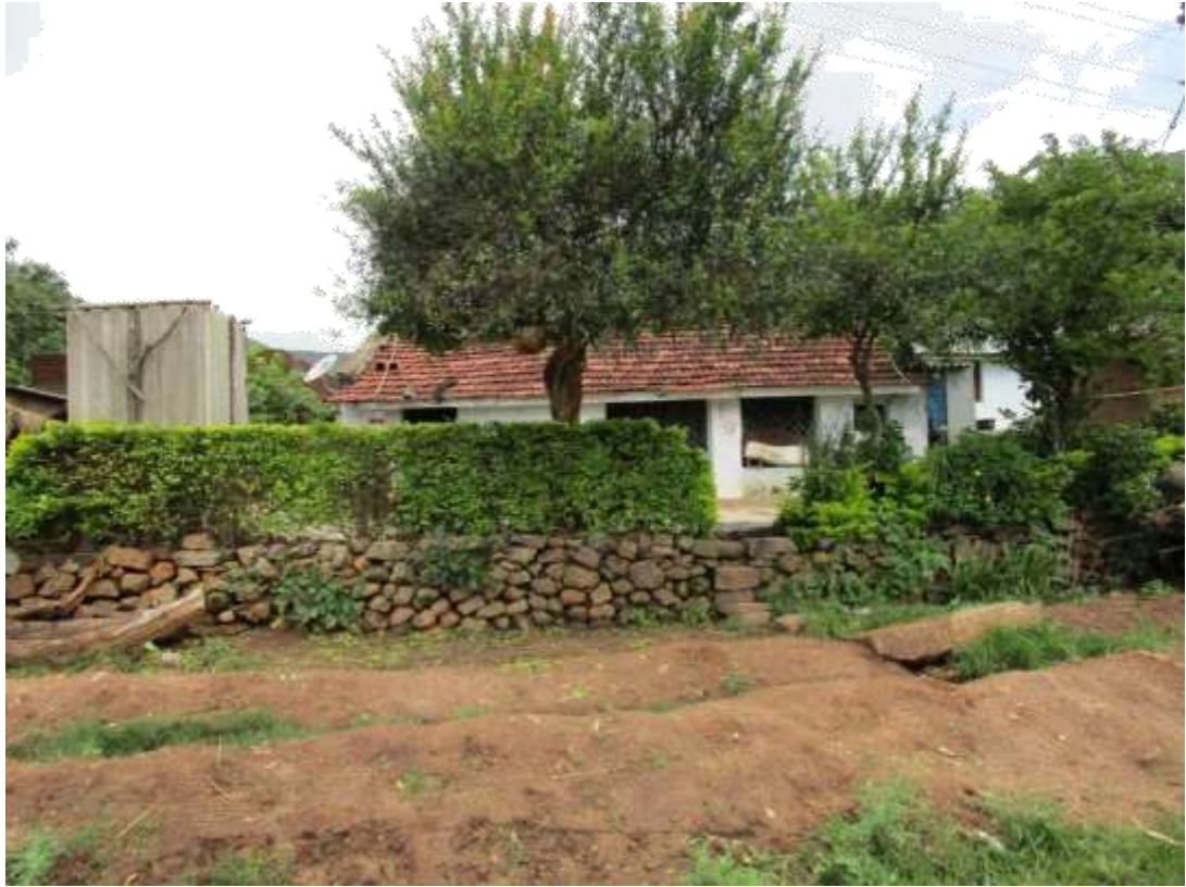
Figure 11 A tiles roofed house with bath room asbestos sheets enclosed by asbestos sheets at Bakuru village, HukumpetMandal
