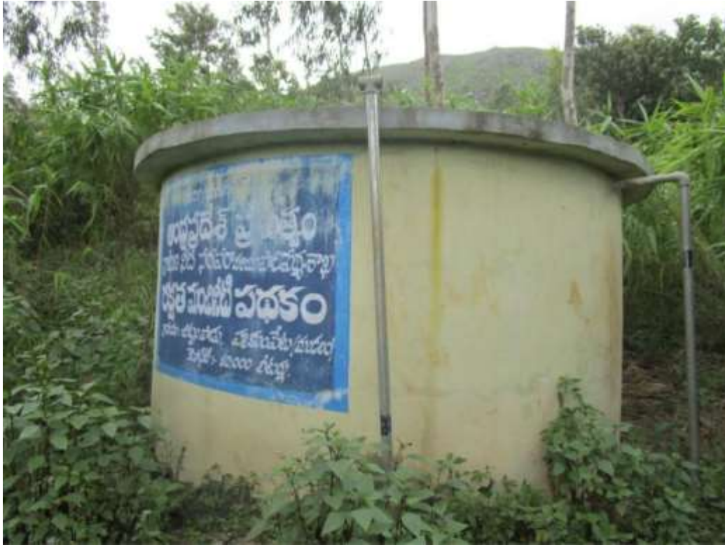
Figure 53 Protected drinking water tank in Chittampadu village, HukumpetMandal
