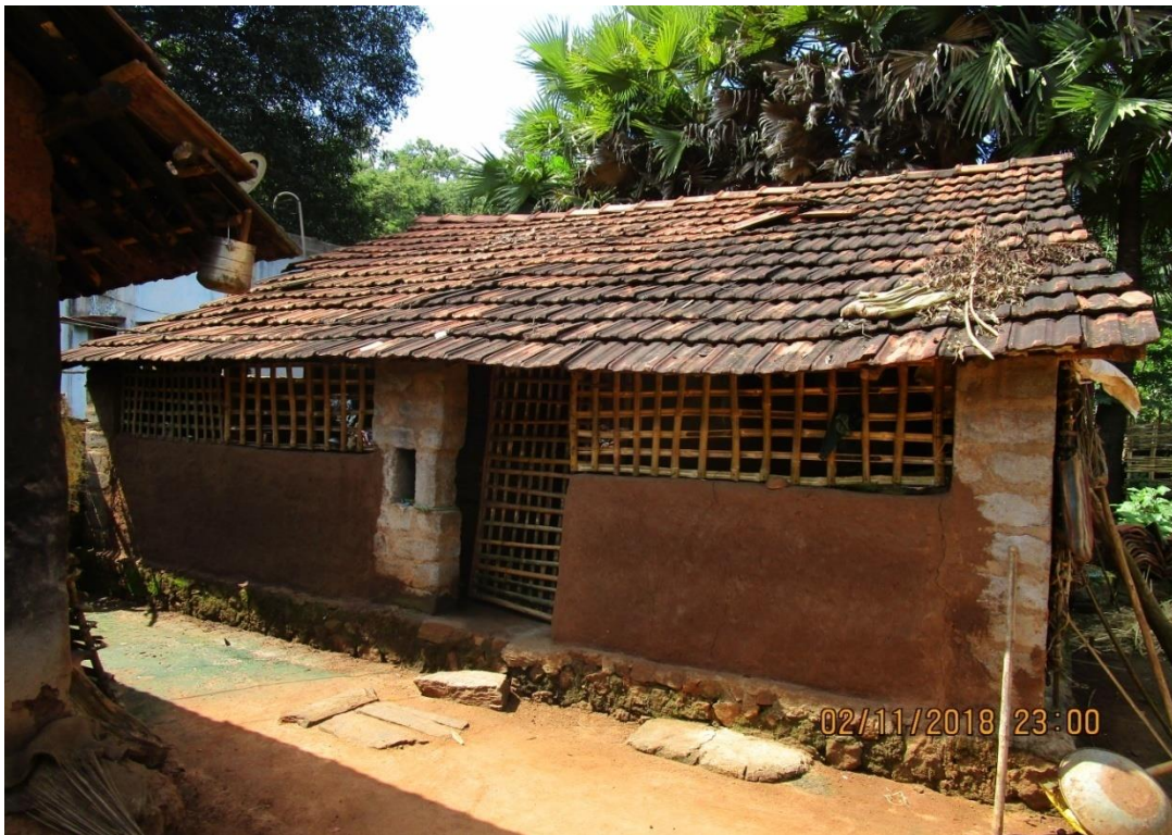
A tile roofed house of Konda Kapu with mud walls in Rampachodavaram ITDA, East Godavari dist
