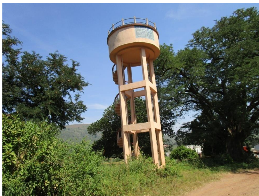
Over head drinking water tank at Kuridi village, Paderu ITDA, Visakhapatnam, dist
