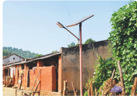
Installation of Solar light system Vill-Madalakuna, G.P-Belghar, Block-Tumudibandha, Dist-Kandhamal under CCD Plan 2009-10
