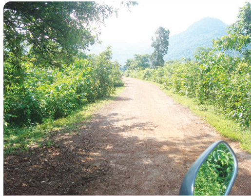
C.D. work and C.C. Road from Purunaguma to Oringi No. of beneficiaries - 120 nos.
