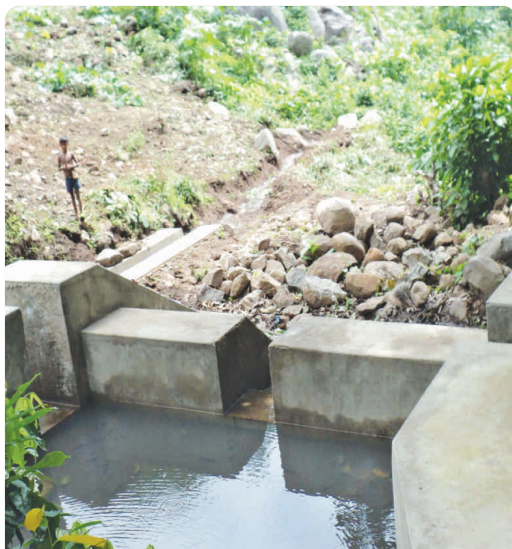
SCA TO TSP Check Dam at Maisingkhatanala at Ramakasahi, Chandragiri
