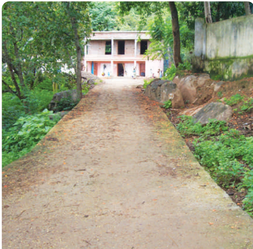
Const. of C.C.Road with Culvert from R.D.Road to MPSC Building at Sagoda through SCA TO TSP 2009-10
