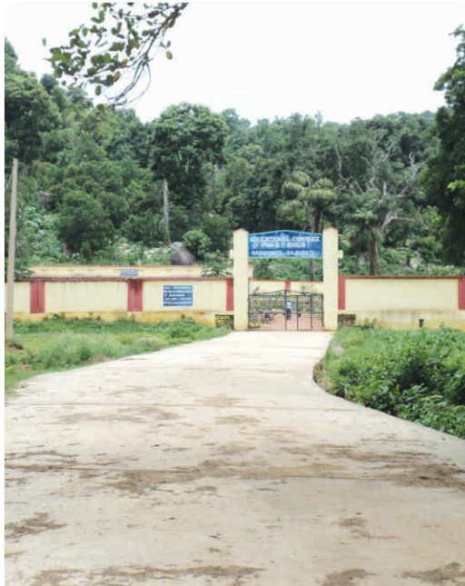
Approach road (CC Road) to Education complex at Baghamari, Chandragiri constructed under CCD Plan
