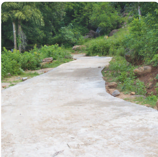
Construction of C.C.Road from G.P.Road to Kurudi MPSC Building thorough SCA TO TSP 2009-10
