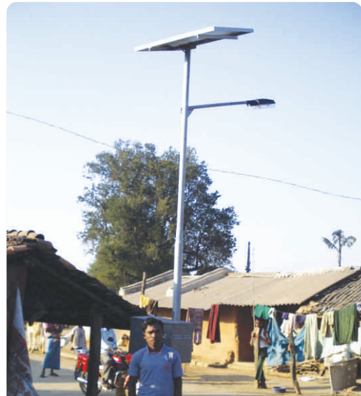
Solar Street Light at Kopaguda Village
